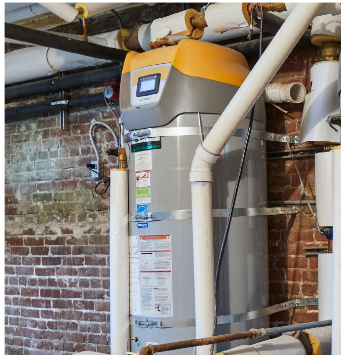
A heat pump water heater installed in a Bay Area property.
