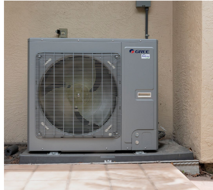
Heat pump condenser.
