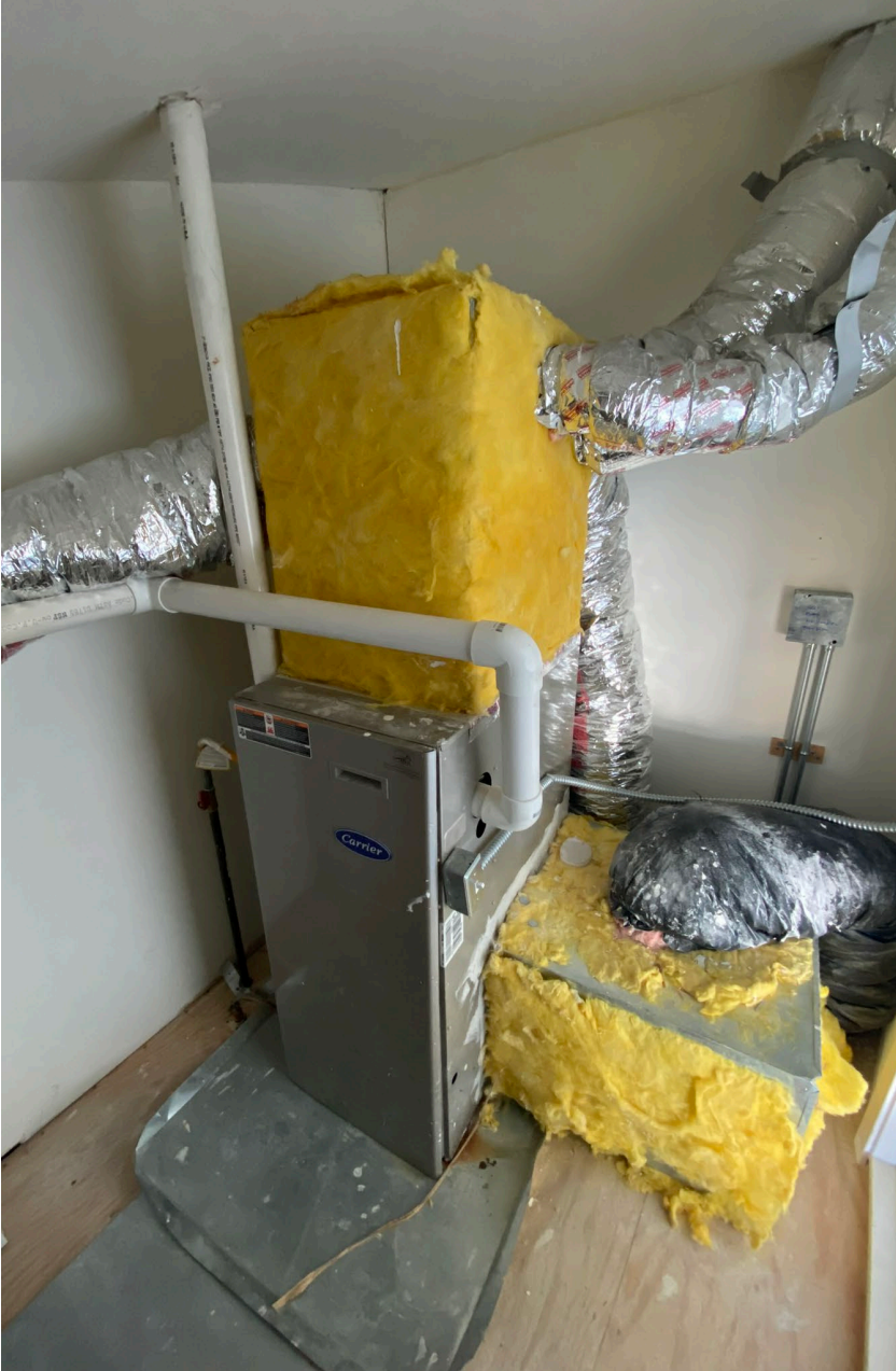
Old furnace in attic above closet
