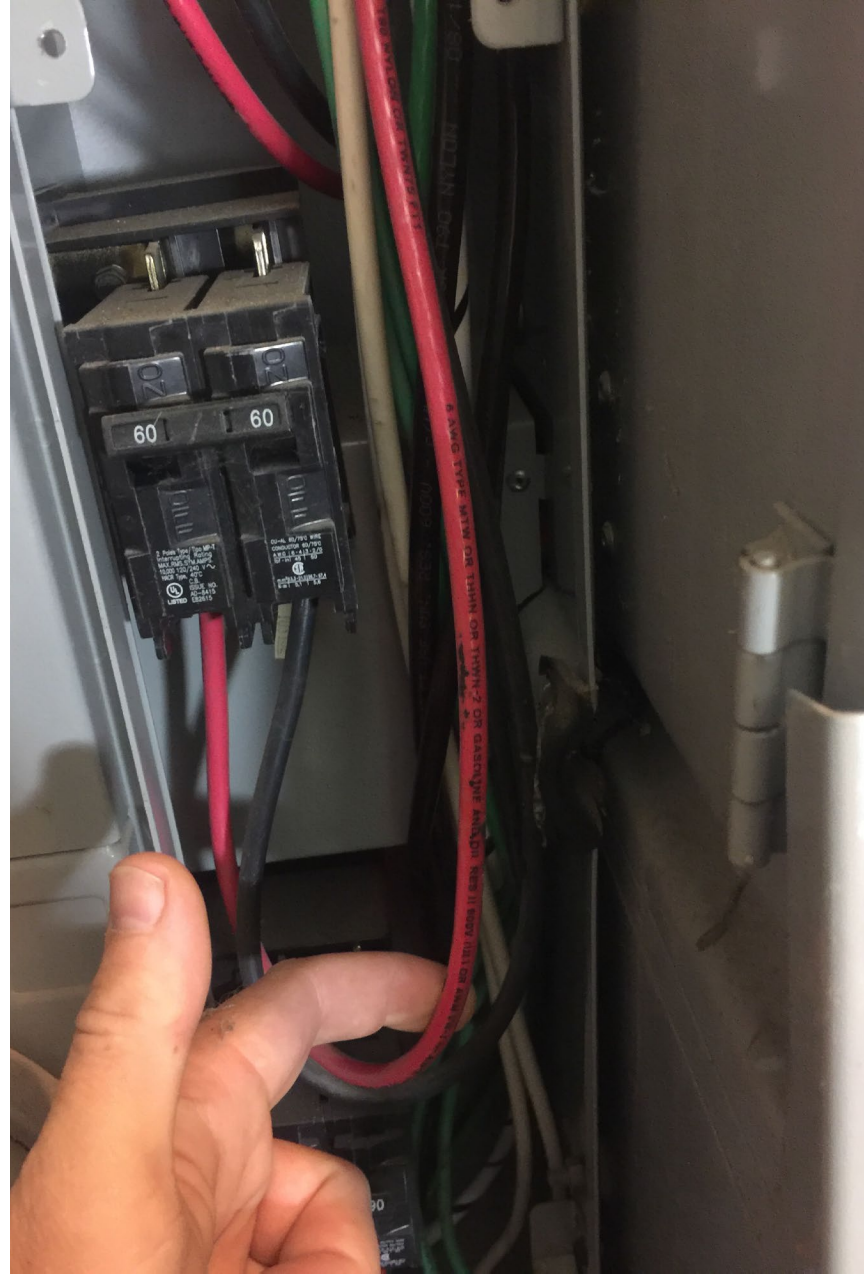
Wiring not torqued
