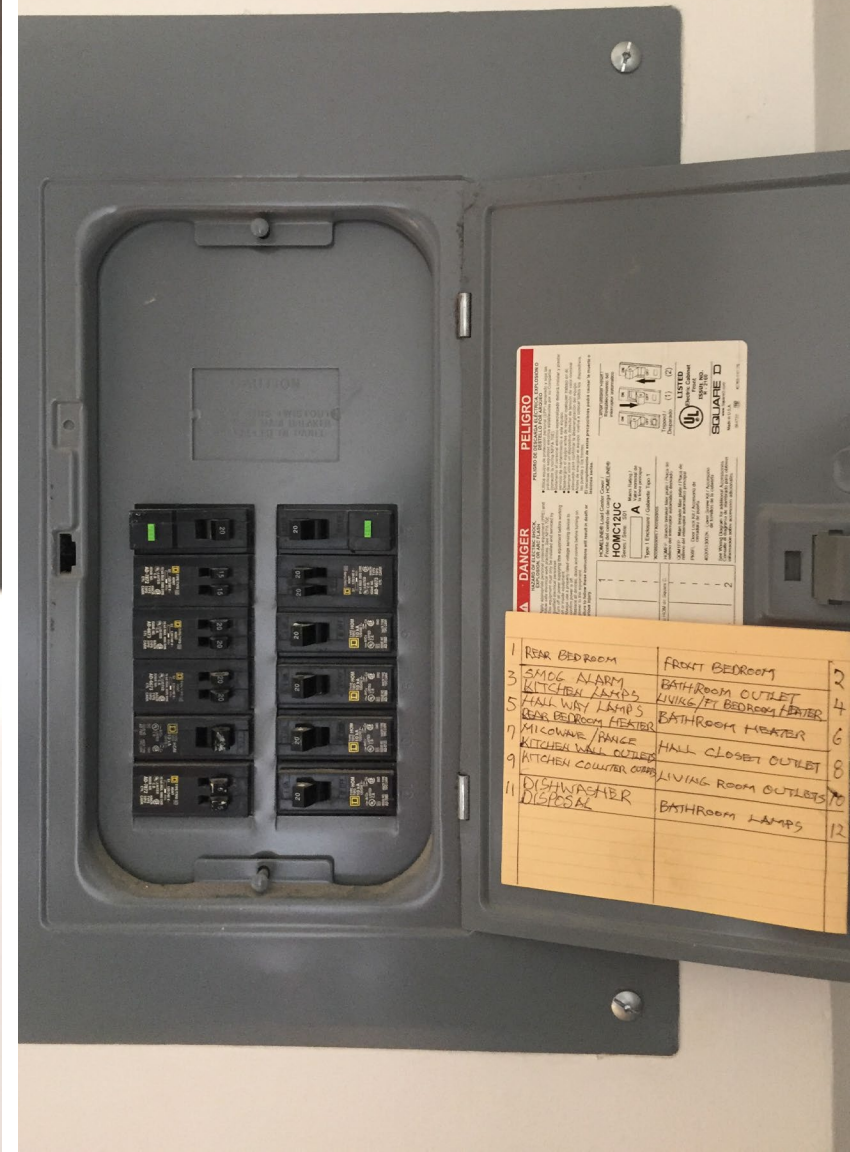
Full subpanel in unit
