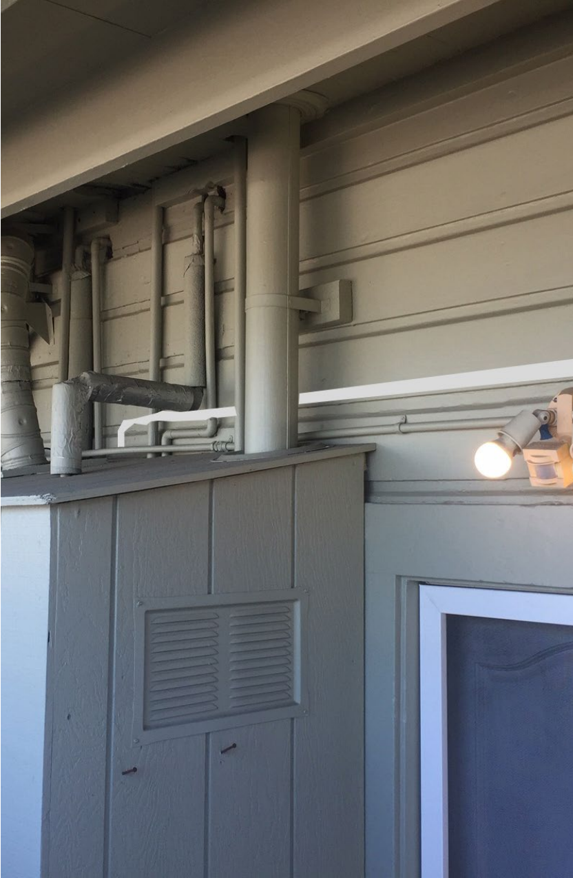
Landing water heater closet
