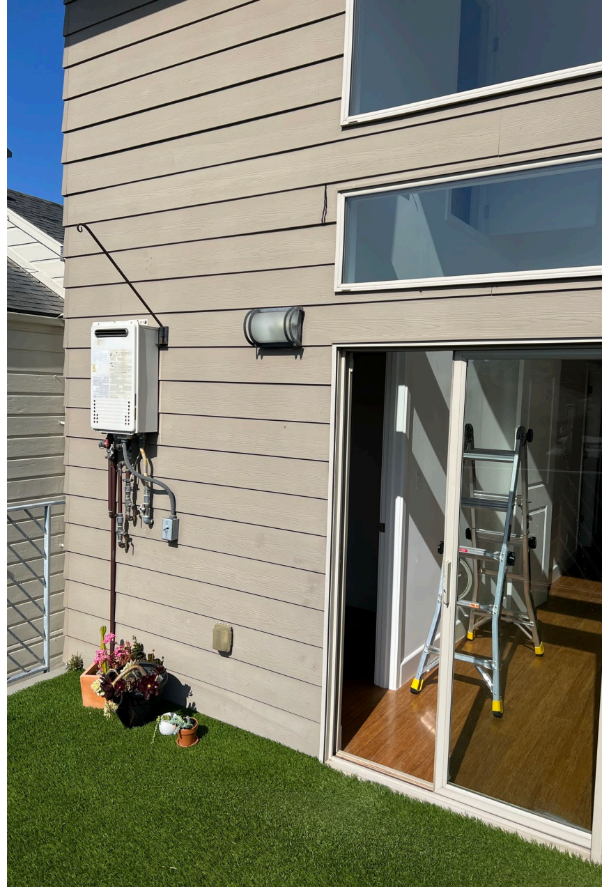
Back deck on-demand water heater
