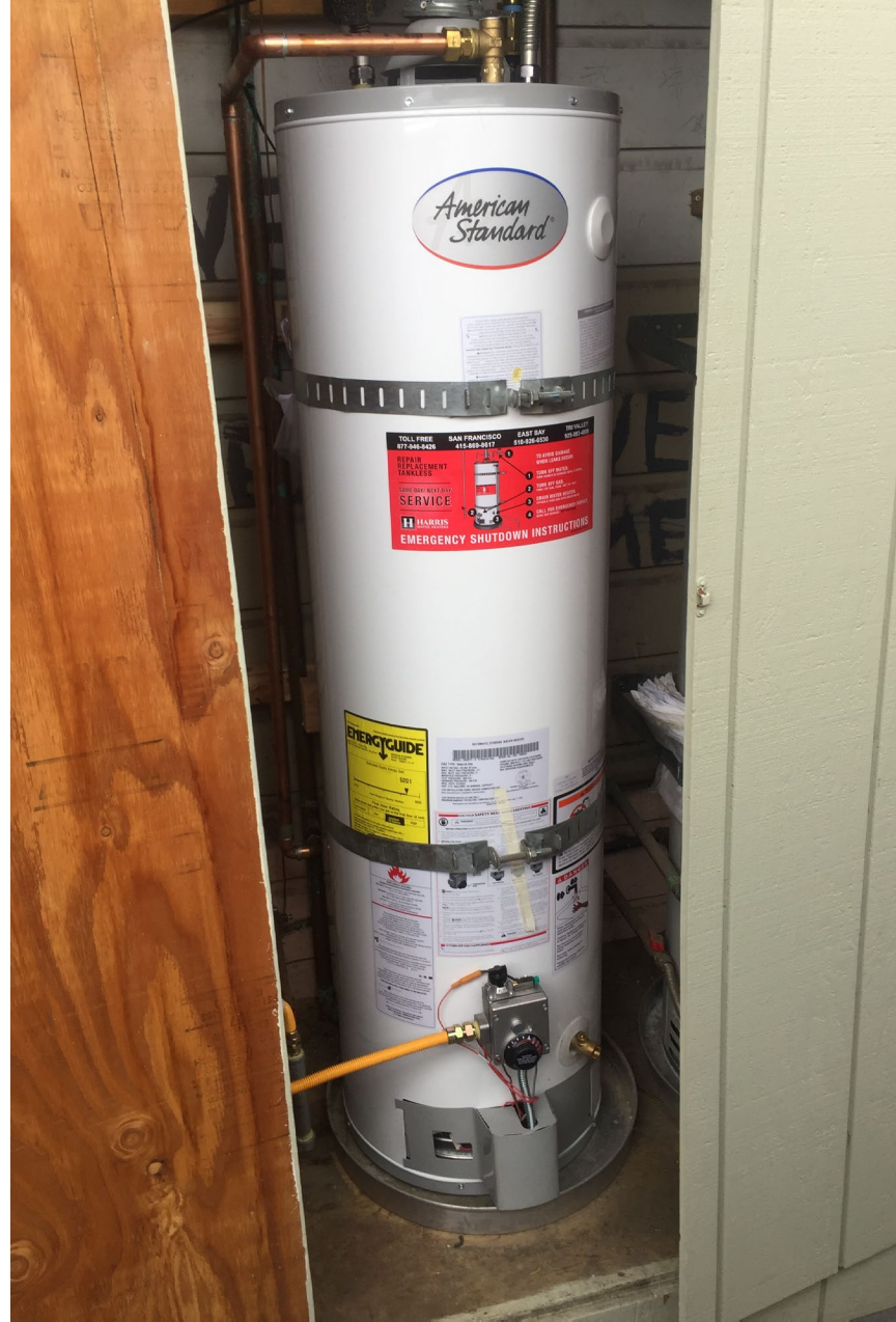
Gas water heater
