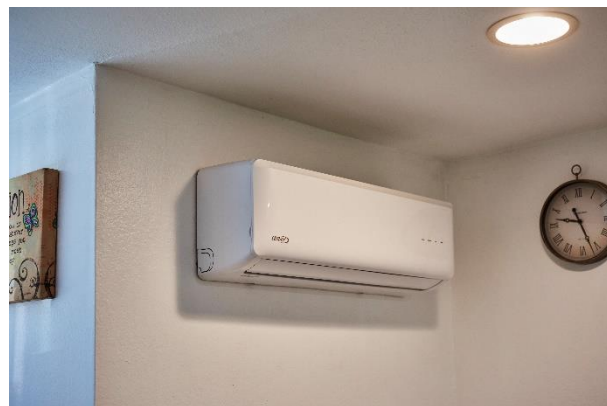
A newly installed ductless mini-split heat pump, which provides residents with heating and cooling
