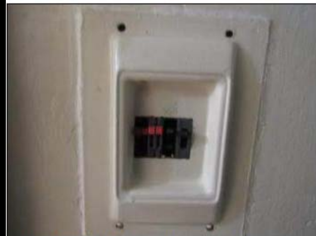
113. Temple I Unit Circuit Breaker Panel
