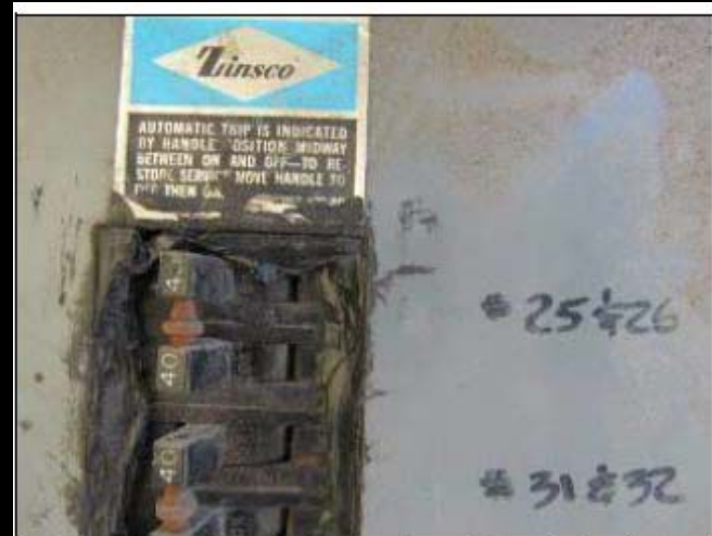
111. 40-amp 2-pole 40-amp 2-pole Circuit Breakers
